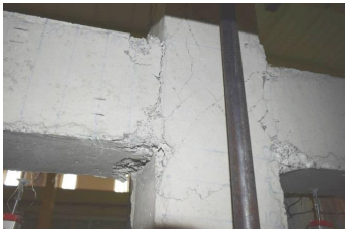
Figure 12. Crack development in SAMPLE1
