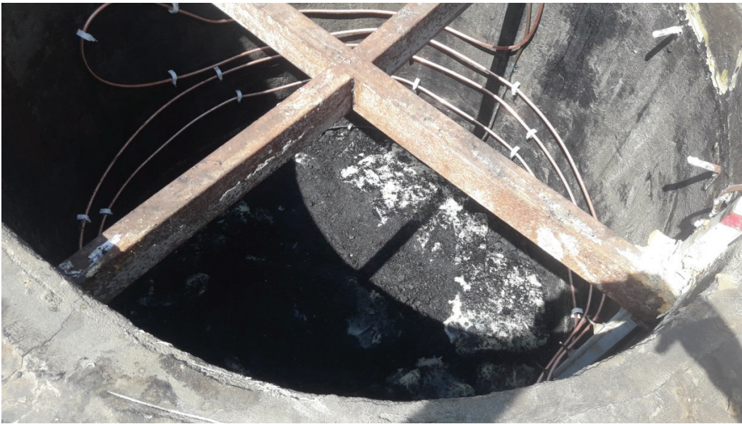
Figure 7. A Picture of the experimental unit after the removal of water and wet coal and the installation of the second heat exchanger (copper coil). The experimental unit was constructed at the city of Nasiriya-south of Iraq and had three layers, a layer of paraffin wax with a thickness of 10 cm, a layer of coal with a thickness of 30 cm and a gap of air with 80 cm depth.
