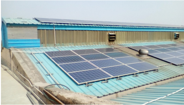
Figure 1. View of 227 kW installed roof top power plant.
