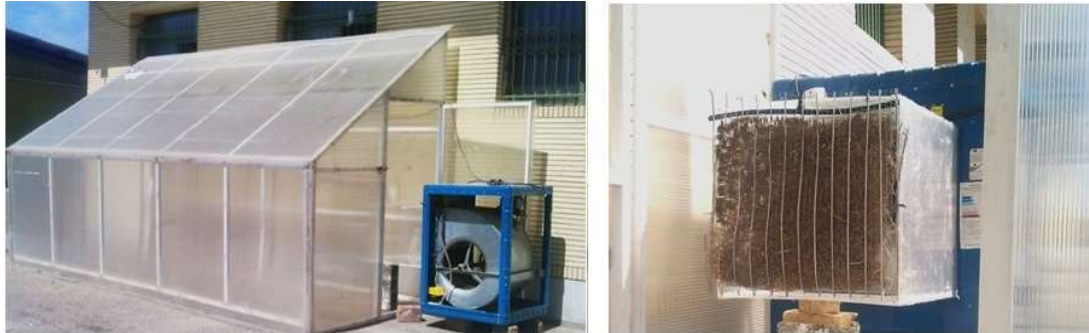
Figure 3. Photographs of the greenhouse and the evaporative cooling system
