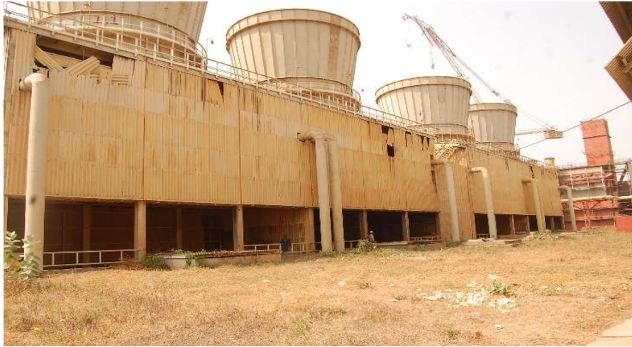
Figure 3. A pictorial view of the arrangement of cooling towers in Ajaokuta Steel Rolling Mill
