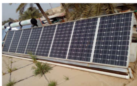
Figure 3. Part of the PV system used in ERET
