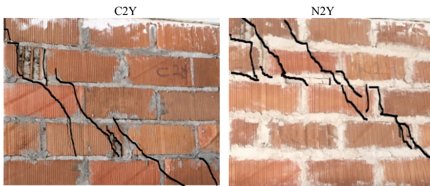
Figure 4. Damage of the Walls produced with Masonry Brick
