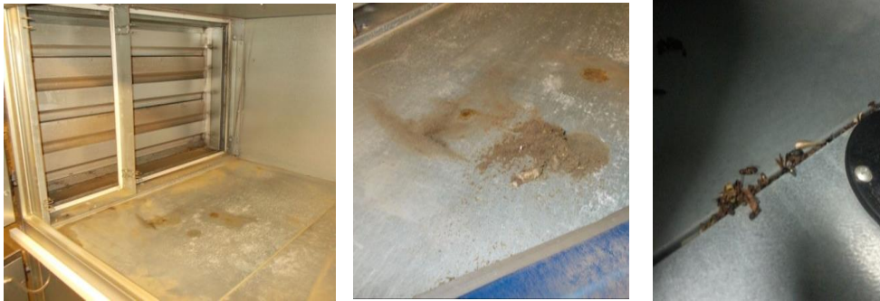
Figure 9. Demonstration of pollution of the filter chamber on the side of the intake of fresh air (left), solids trapped in the joint between the panels (right)
