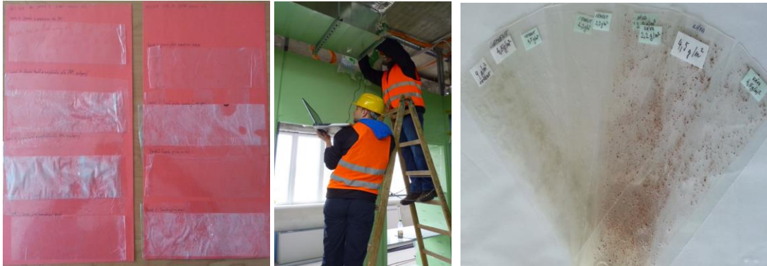
Figure 5. Example of assessment of pipework contamination by visual inspection using checking benchmark method (right), the samples (left)
