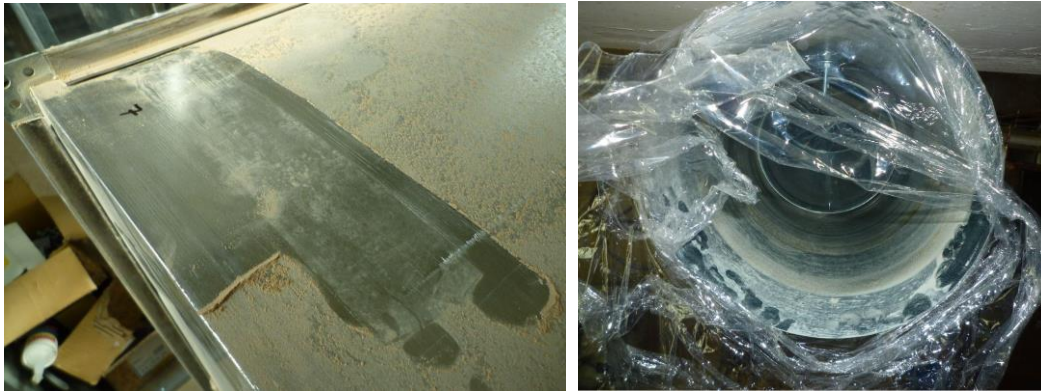
Figure 1. Sample contamination during ducts assembly (on the outside – left, on the inside - right)
